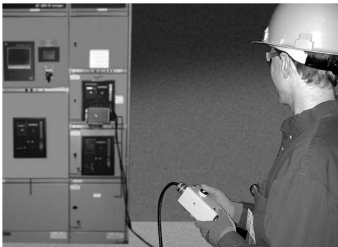
Figure 4.1 Remote Racking Operation
